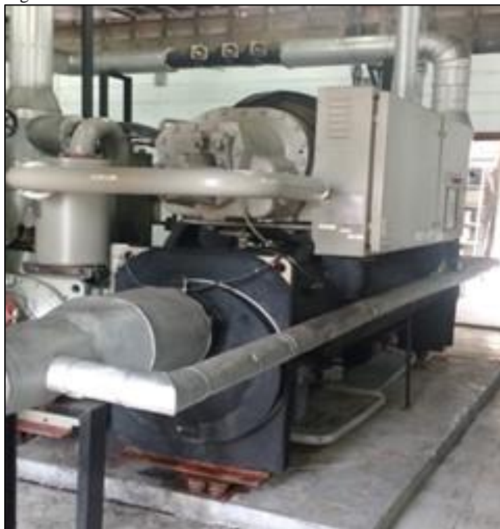
Figura 14 – Chiller RTHC 300TR
