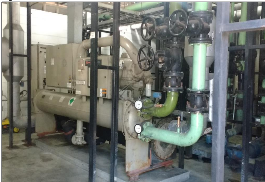
Figura 15 – Chiller RTHC 215TR
