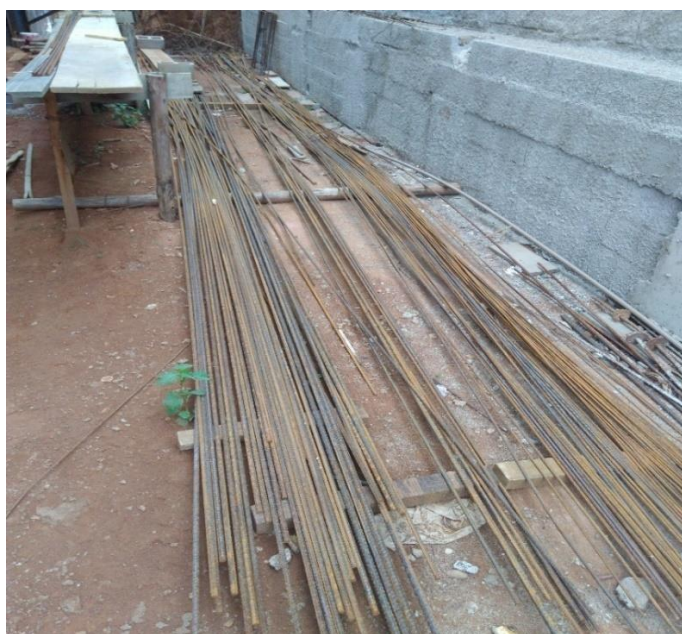
Figura 16: Barras de aço expostas as intempéries.
